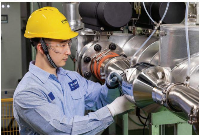
In 2023, BASF inaugurated a new Maintenance Repair and Overhaul (MRO) Station in Shanghai. A technician is testing an ozone and ozone/VOC converter.
