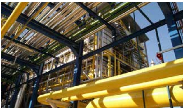
Our pipelines transport steam and products from one plant to another. This way we act responsibly with raw materials and energy
