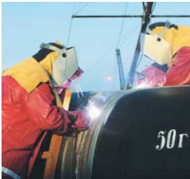
On the Russian mainland, work starts on the North European Gas Pipeline – a joint venture between BASF, Gazprom and E.ON.
