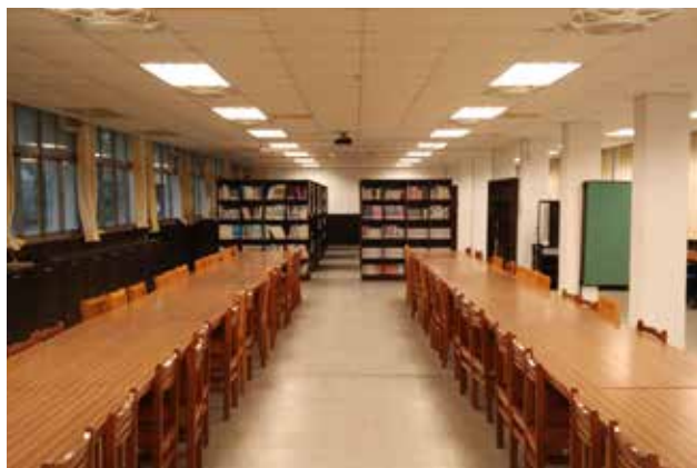
Primary school classrooms after the installation of T8 fluorescent LED lighting tubes using BASF's newly developed color converting technology.
