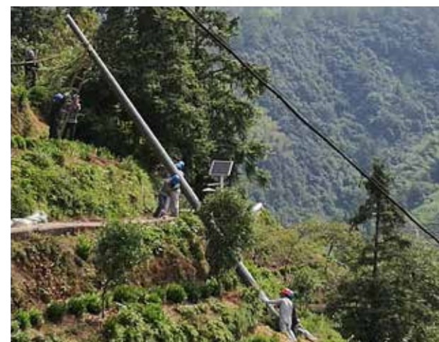
Polyurethane composite utility poles help ensure power supply in China's mountainous regions.
