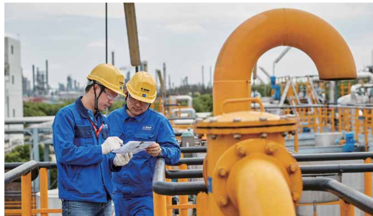
At the tank farm of BASF Polyurethanes Specialties (China) Co. Ltd. in Shanghai, off-gas is treated within the facility and exhausted through the emission point (the yellow curved pipe).
