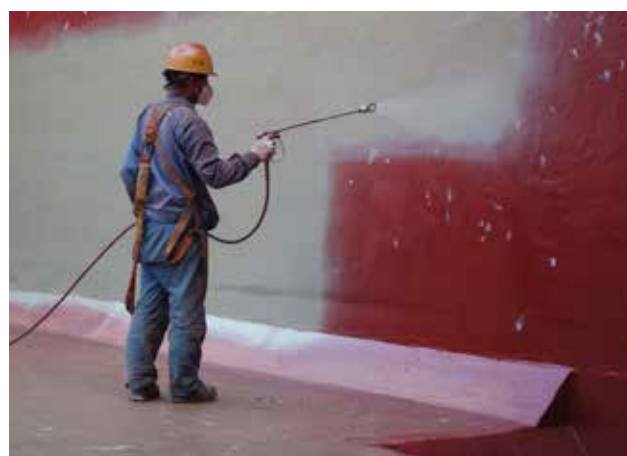
MasterSeal 7000 CR is applied to the sewage tank of Sino French Water's Shanghai plant.
