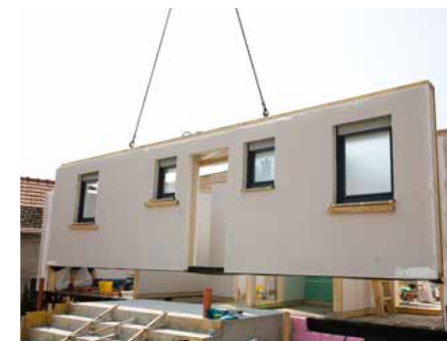
Building prefabrication makes on-site construction more efficient and ensures better quality control of building components.
