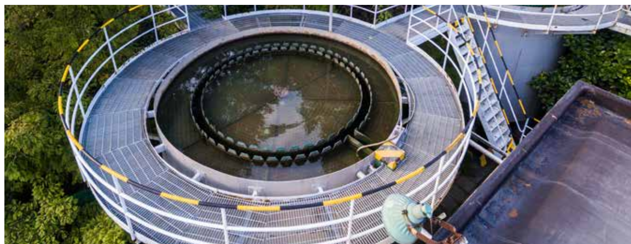
The water station at BASF Shanghai Pudong Innovation Park purifies and filters water from the Huangpu River, before supplying it for purposes of production, cooling and firefighting.
