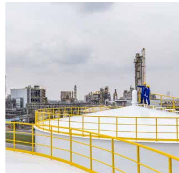
At Shanghai Caojing site, two inspectors conduct a regular check of the water tank for firefighting, ensuring all facilities for emergency response are in the best possible condition.
