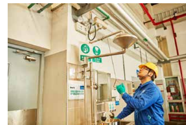
Emergency shower facilities can be found in every plant and laboratory.
