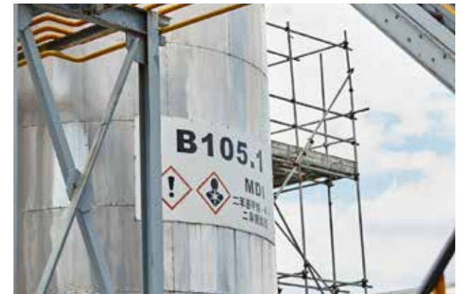
Safety labels on the MDI tank
