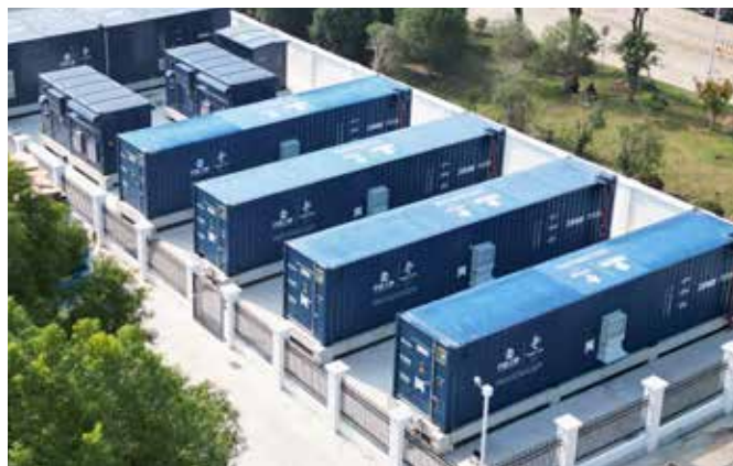
BASF's first power storage station in China went into operation at its Shanghai Pudong Innovation Park in 2022.
