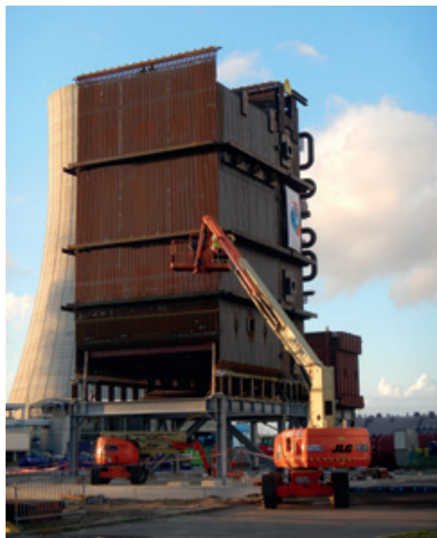
BASF Antwerp is building a steam boiler. This will help anticipating fluctuating energy prices.
