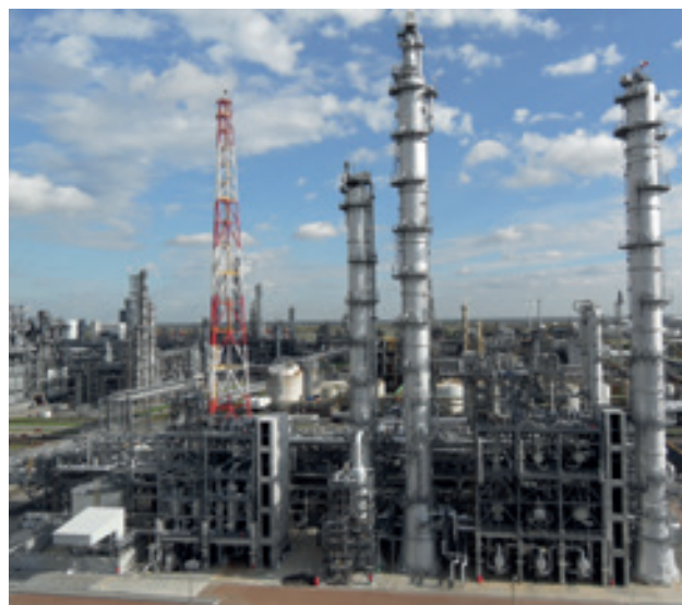
Our butadiene production facility is the most remarkable investment last year.
