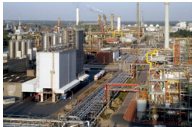
More than 500 km of pipelines ensure that the end product in one plant can be supplied to another plant.
