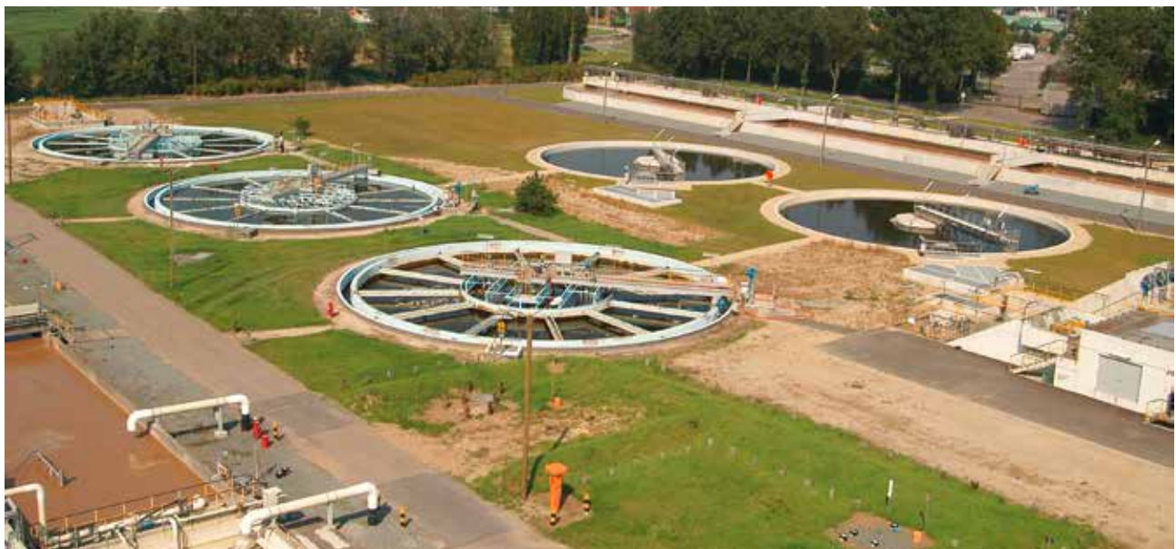
When we took our water treatment plant in use in 1980, we were one of the first companies in the area to biologically treat waste water.
