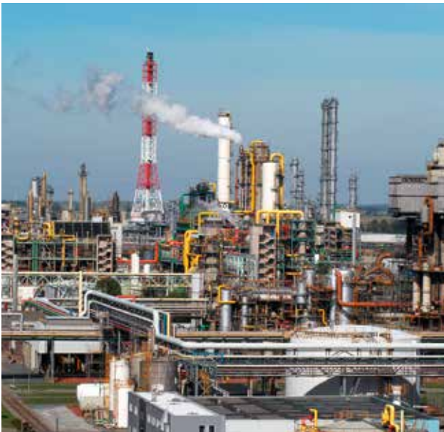
We cover 90% of our thermal needs by a smart steam network, balancing exothermic and endothermic chemical processes.
